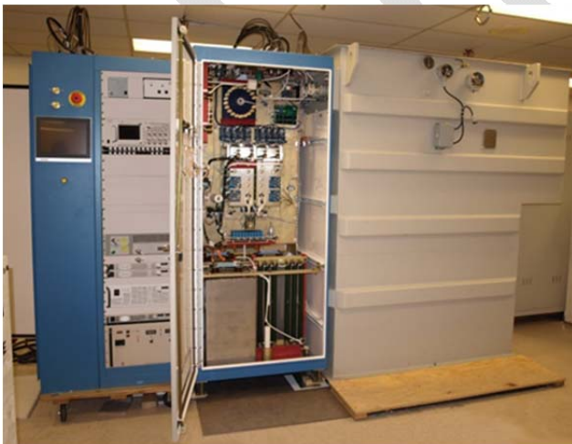
Figure 1. DTI's solid-state ESS klystron modulator. This design is optimized for long pulse operation with highest possible reliability and availability required for particle accelerator user facilities and test stands.
