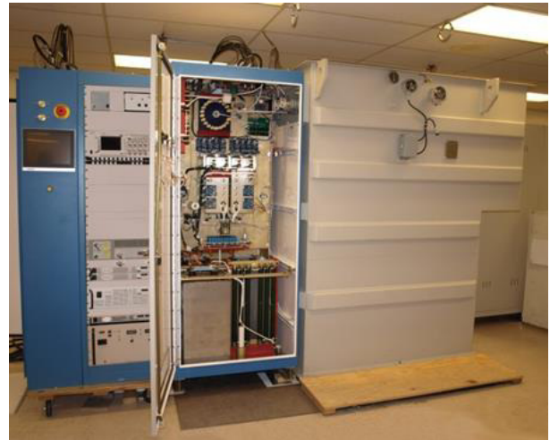
Figure 1: System designed for Oak Ridge National Laboratory Spallation Neutron Source. Design is optimized for long pulse operation with highest possible reliability and availability required for particle accelerator user facilities and test stands. High voltage cables connect to dummy load or klystrons not shown in figure.
