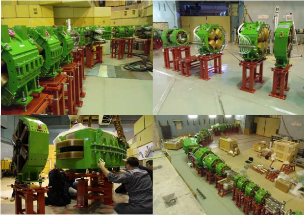
Figure 4: UL Primary beamline, UR 2 quads, 2 6-poles and 1 8-pole in secondary beamline, LL Installation of D1 secondary dipole on its stand, LR End of primary and secondary beamlines with vacuum elements assembled.
