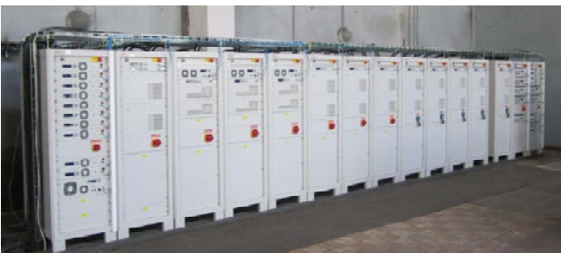
Figure 6: The power supply cabinets.
